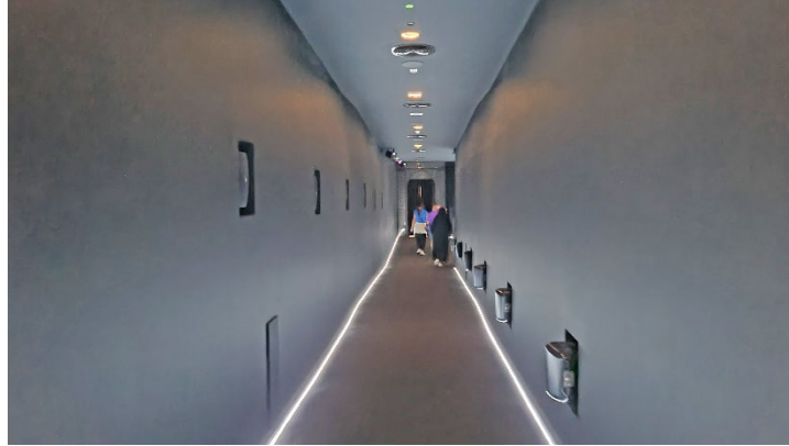
Figure 10. Lighting strips close to the floor surface for enhanced wayfinding
